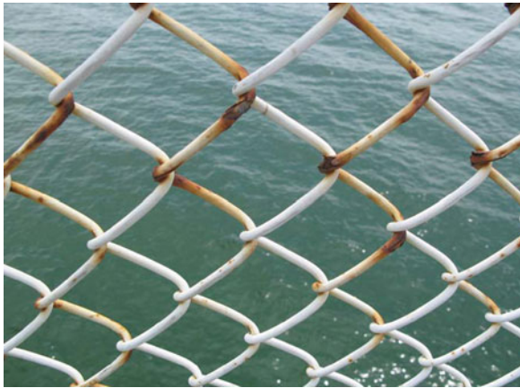
Fig. 12.48 Higher stress regions (and more plastic deformation) occur at the crossover bending points of this chain-link fence. Note the enhanced corrosion rates at these crossover/bent-wire locations. Also note that for each bend, the top surface (in tension) generally shows more corrosion than does the underneath surface (in compression).
