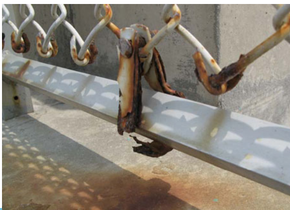
Fig. 12.42 Corrosion failure of a U-type metal support clamp. The metal at the bottom of the support clamp has corroded away. One should note that the corrosion rate was greatest in the regions where the metal was severely bent.
